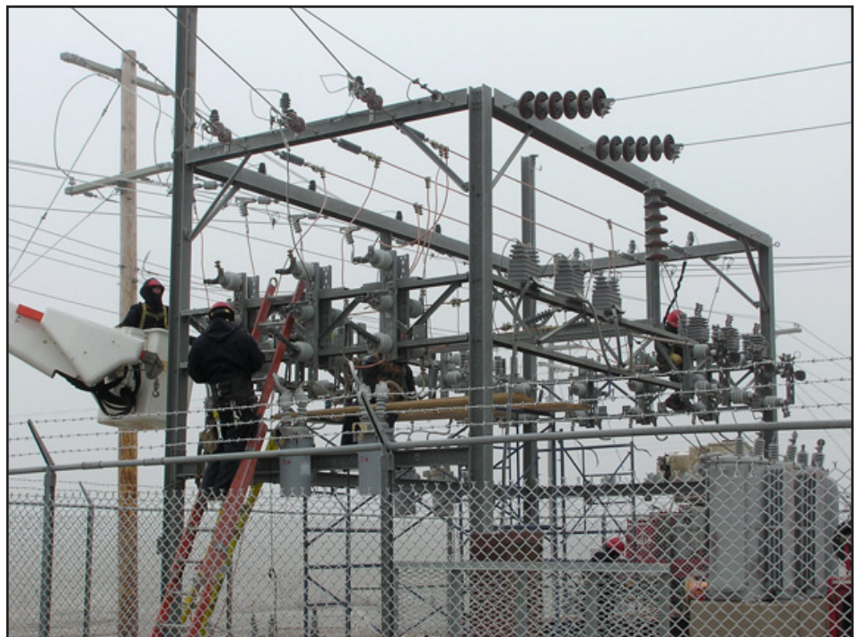
Pictured above are line crews upgrading infrastructure in preparation for transformer upgrade.
