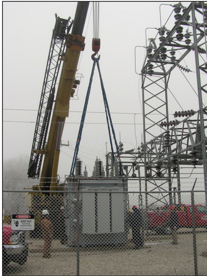
The 3 phase 7.5 MVA transformer weighing in at 49,000 pounds was set into place and installed on December 8, 2010 in the Creighton Substation 85-1.
